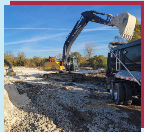
Contractors remove lime at an average annual cost over $250,000.00
