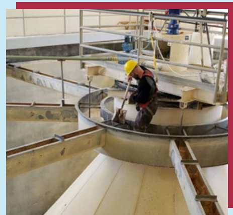
Regular cleaning and parts replacement each year.
