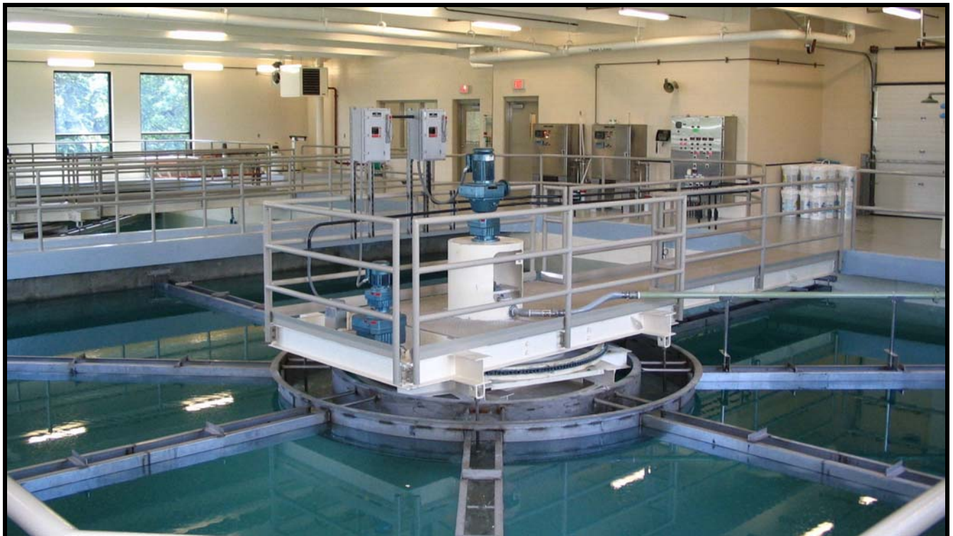
New lime softening clarifiers, part of a $4.8 million water treatment plant improvement project, were fully operational in April, 2004.
