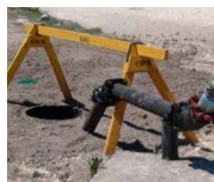
Sludge discharge adapter installed by DPW at the WTP
