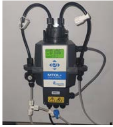
One of four New filter turbidity units
