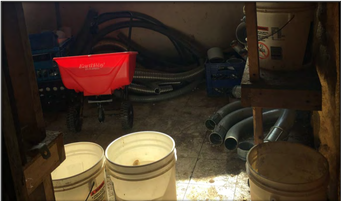
PHOTO: 2 DATE: 2/22/2019 BY: Greg Ross SUBJECT: HA 4: Asbestos-containing 9x9-inch floor tile located in the storage area (with shower), south of Ludington Electric's shop.
