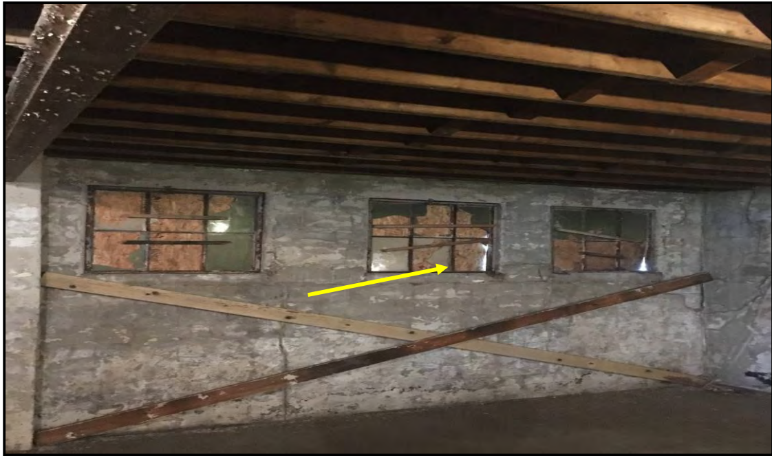
PHOTO: 1 DATE: 2/22/2019 BY: Greg Ross SUBJECT: HA 1: Asbestos-containing glazing on the metal frame windows located in the eastern portion of the building on the second floor (10 windows total).
